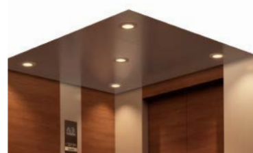
Ceiling: L210S LED downlights (yellow-orange)
